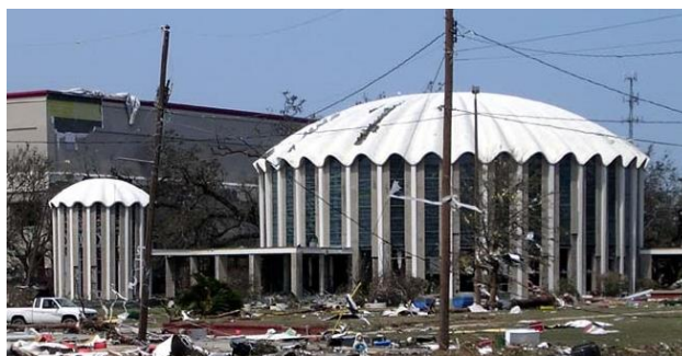
Figure 5. Damage to the scalloped dome roof of St. Michael's church in Mississippi because of Hurricane Katrina
