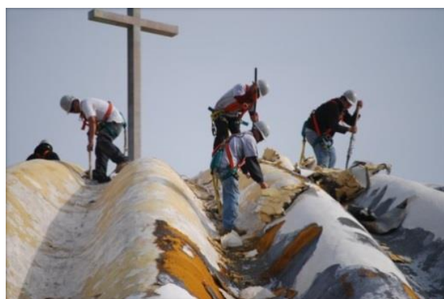
Figure 6. Damage to the scalloped dome roof of St. Michael's church in Mississippi because of Hurricane Katrina
